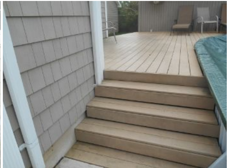
Missing handrails. Rec. handrail installation. Safety concern.
