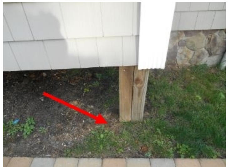
4x4 wood support in contact with ground, this can lead to wood rot & pest infestation. Rec. licensed contractor to fix.
