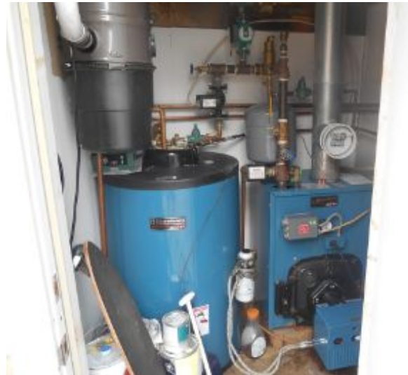
Utility room with boiler, water heater & central vac unit.
