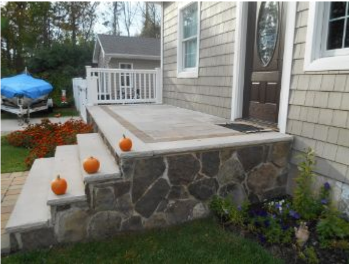
No handrails noted, safety concern. Recommend placing hand rails.
