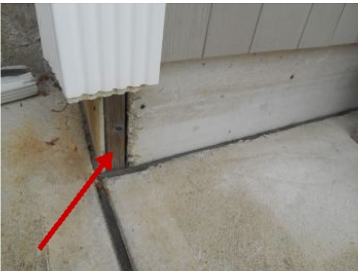
Exposed framing, can lead to water infiltration & wood rot. Rec. licensed contractor.
