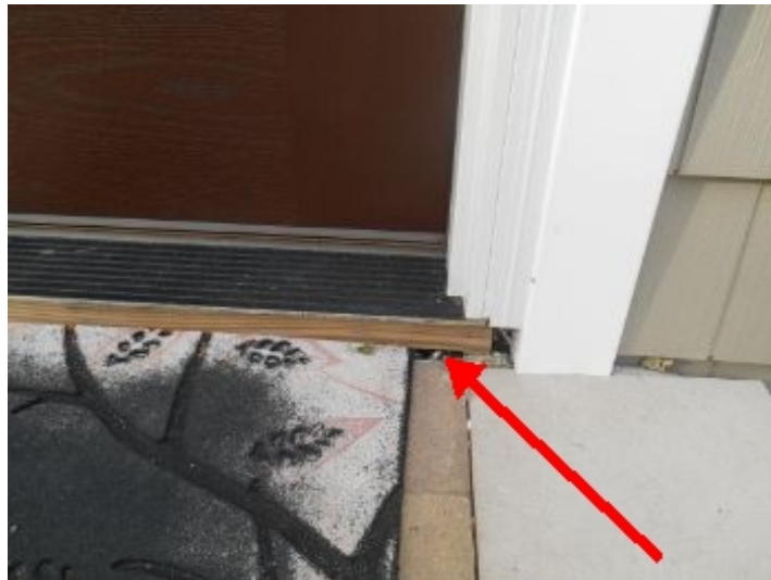
Front door sill missing flashing. Will lead to water infiltration. Rec. licensed contractor.
